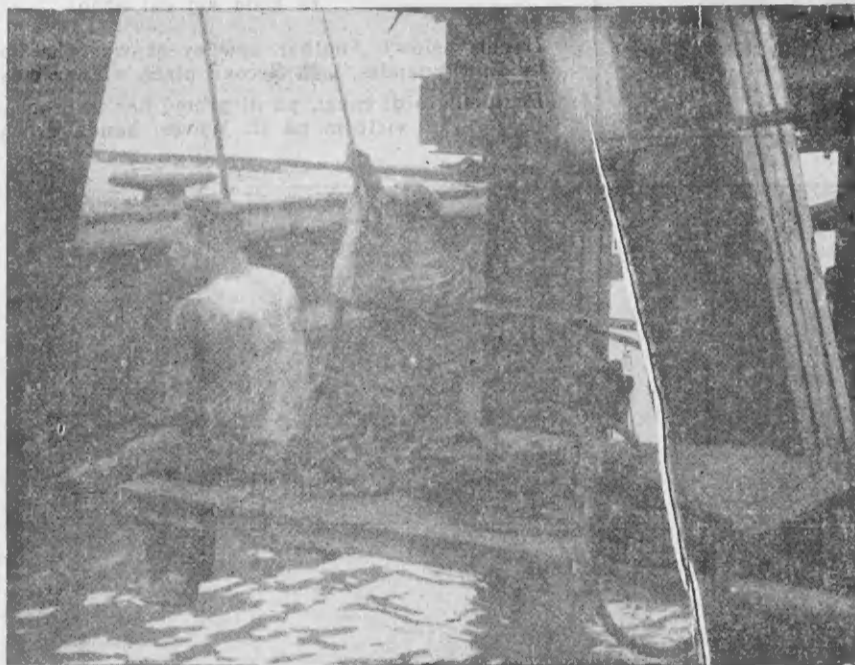
An important day for Aruba and Lago. The last pile of the big new No. 2 Finger Pier is driven, marking a vital point in the construction of the pier. Two Netherlands Harbor Works men manipulate the ropes which control the hammer of the pile driver, "Aruba".
